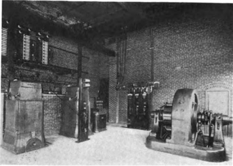
INTERIOR CHASELAND SUB-STATION, COLUMBUS, DELAWARE & MARION
